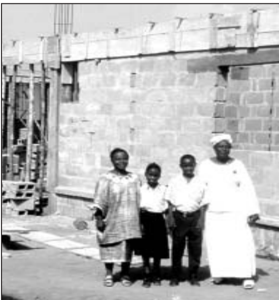
▲ Built with Holston Funds: Principal Ruth Doe and Vice Principal Mary Bedell stand with two students in front of the 'Holston Conference Building,' a new two-story addition to the J.J. Roberts School.
