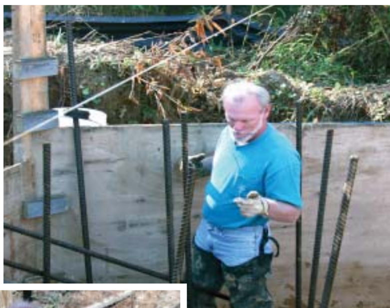
Harry Howe builds a bridge for four needy families near Nebo, Va. He has written a poem, "She Sits Alone," that captures his commitment to construction ministry. To read the poem, visit www.holston.org/thecall .
